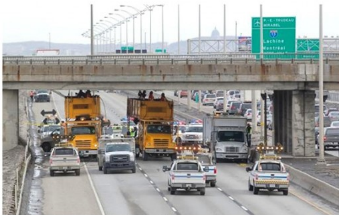
Photographs by: Phil Carpenter, The Gazette
